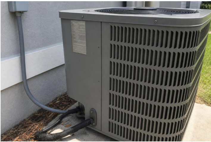
HVAC system photos - HVAC system photos
