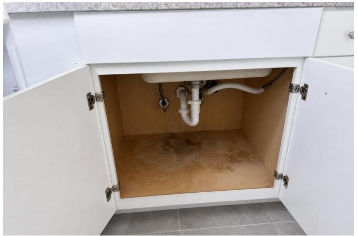
Plumbing system photos - Plumbing system photos
