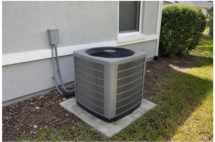
HVAC system photos - Exterior condenser in serviceable condition.
