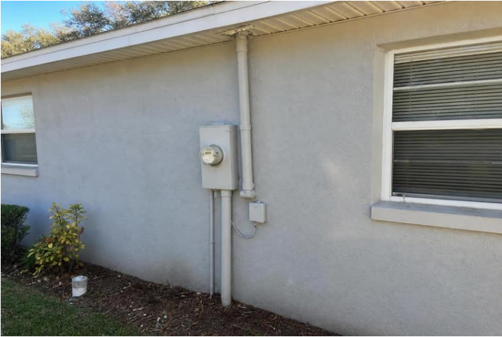
Additional photos - Additional context photo for noted minor deficiencies.
