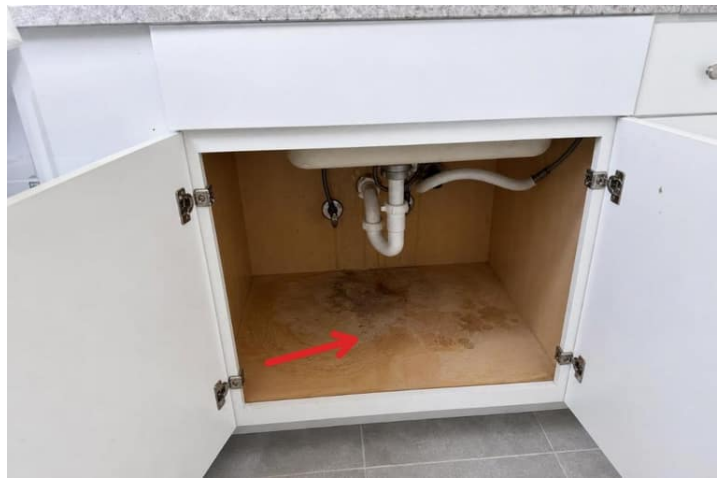
Plumbing system photos
