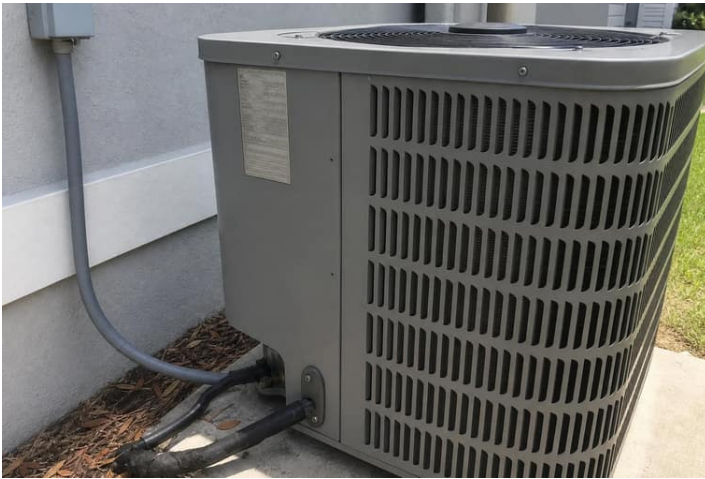
HVAC system photos - HVAC equipment and data plate area; 2019 manufacture year.
