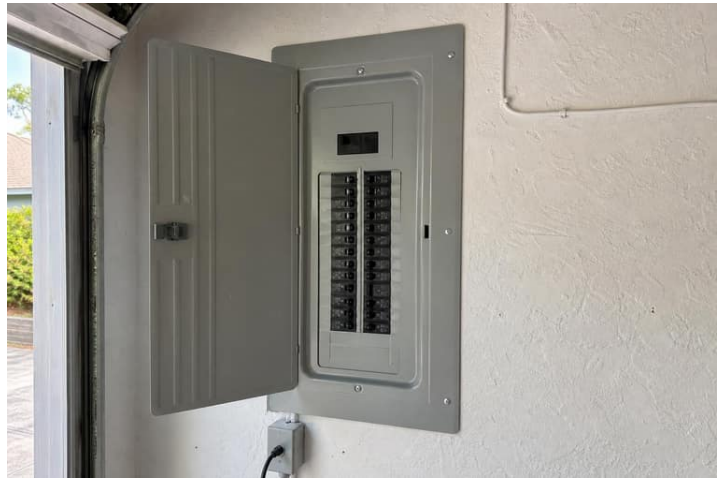
Electrical system photos - Main panel overview; 150-amp circuit breaker panel.
