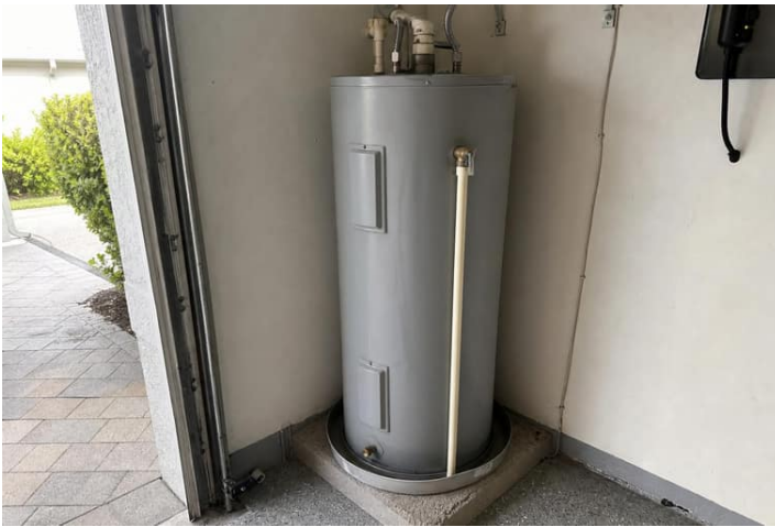
Plumbing system photos - Garage water heater with TPR valve present; satisfactory condition.
