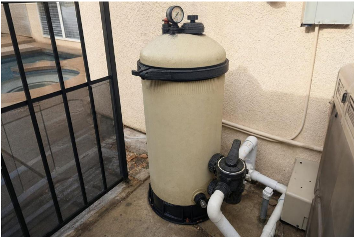
Pump, Filtration, and Plumbing 6.2a - Filter tank and filter components
