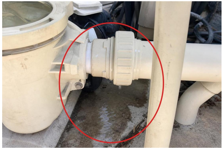
Pump, Filtration, and Plumbing 6.1b - Pump operation and visible condition
