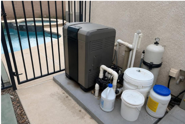
Heater and Heating Equipment 7.1a - Heater visible condition and installation
