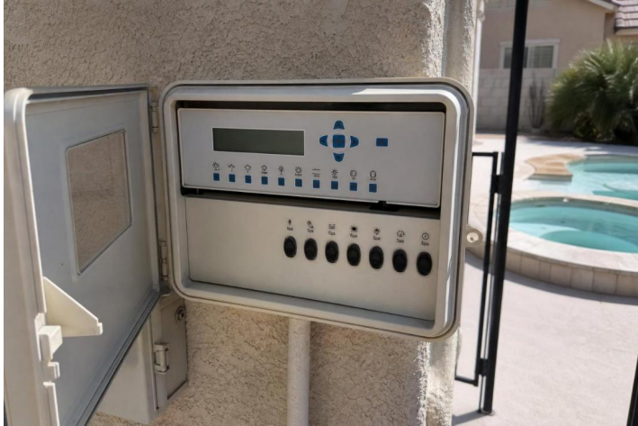
Electrical, Lighting, and Bonding 8.3a - Lights and controls observed
