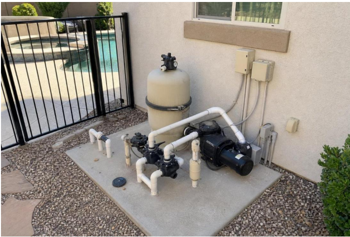
Pump, Filtration, and Plumbing 6.1a - Pump operation and visible condition
