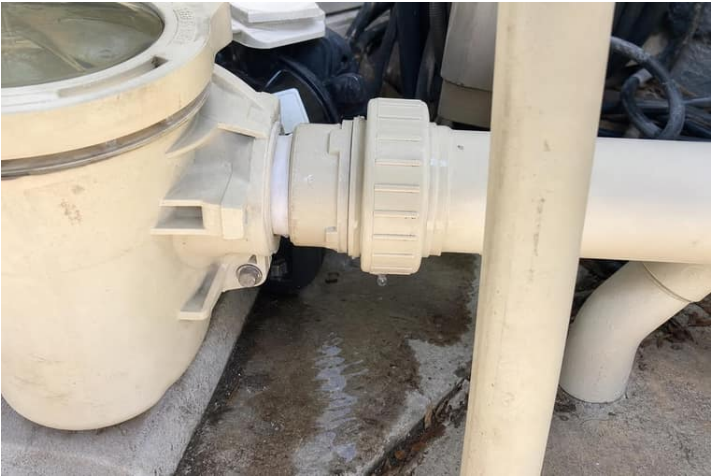
Pump, Filtration, and Plumbing 6.1b - Close view of pump union area where minor dripping was observed.
