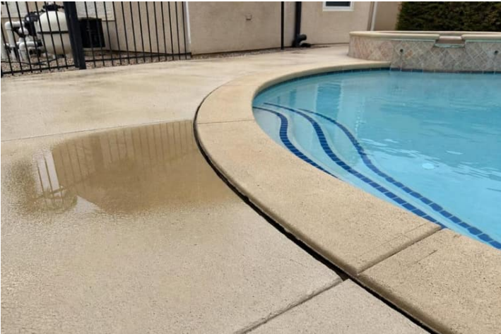
Deck and Access 2.5a - Deck separation and minimum safety standards
