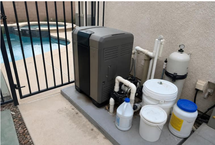
Heater and Heating Equipment 7.1a - Pool heater visible condition and clearance area.
