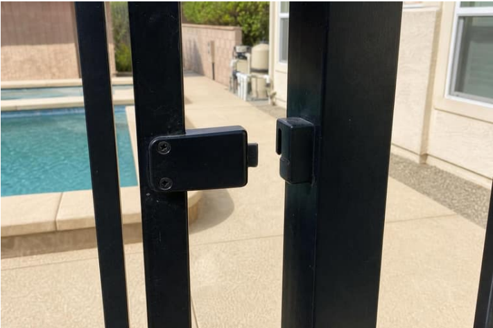
Safety Barriers and Devices 9.2b - Gate latch alignment gap after the gate failed to self-latch.
