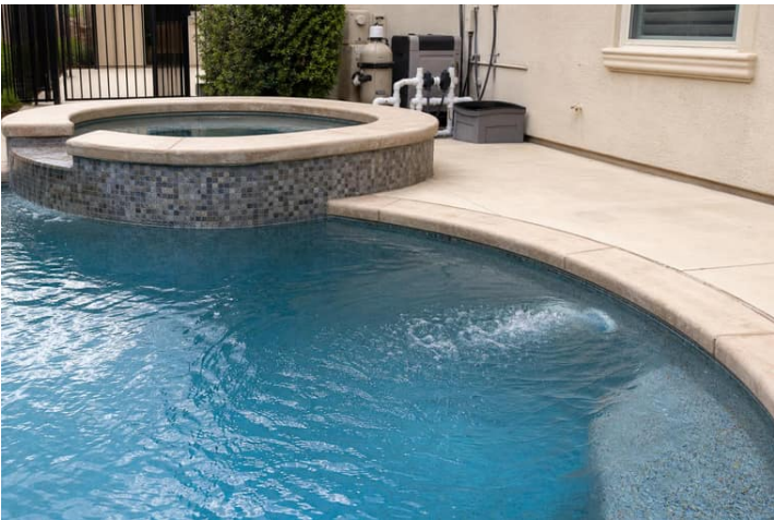
Water Flow and Circulation 3.1a - Return flow observed during basic circulation check.
