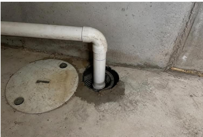
Drain-Tile, Sump, And Suction Points 2.2a - Drain control location where a one-way valve was not observed.
