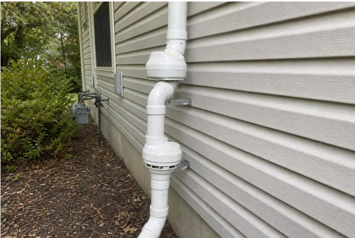
Vent Piping, Fittings, And Supports 4.6a - Exterior piping material and visible marking condition.
