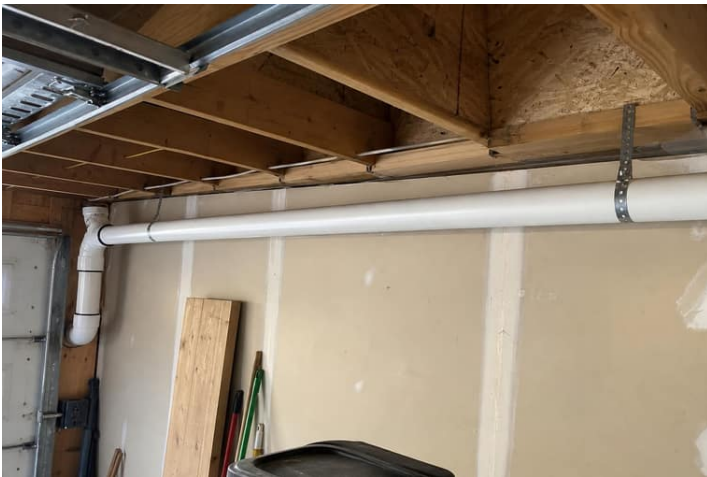
Vent Piping, Fittings, And Supports 4.3a - Horizontal piping support spacing concern.
