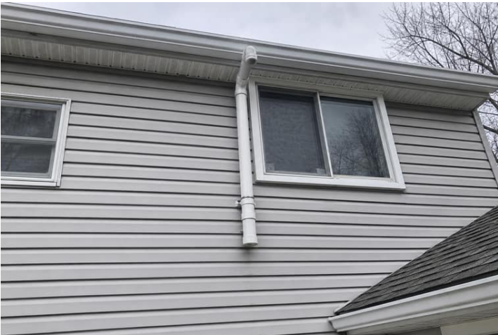
Radon Fan And Discharge 5.3a - Discharge termination near an upper-level window.
