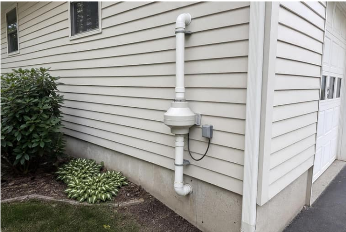
Radon Fan And Discharge 5.1a - Exterior radon fan mounting and visible installation.
