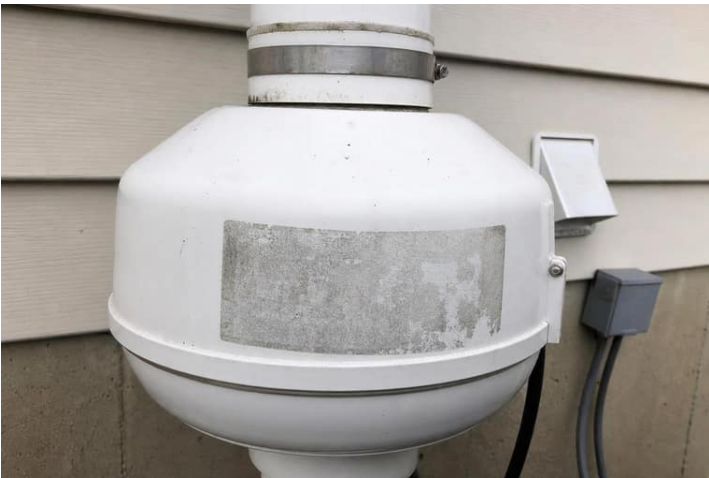
Radon Fan And Discharge 5.2a - Weathered fan label where rating was not verified.
