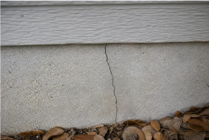
Close detail of the hairline slab crack showing minimal surface separation.
