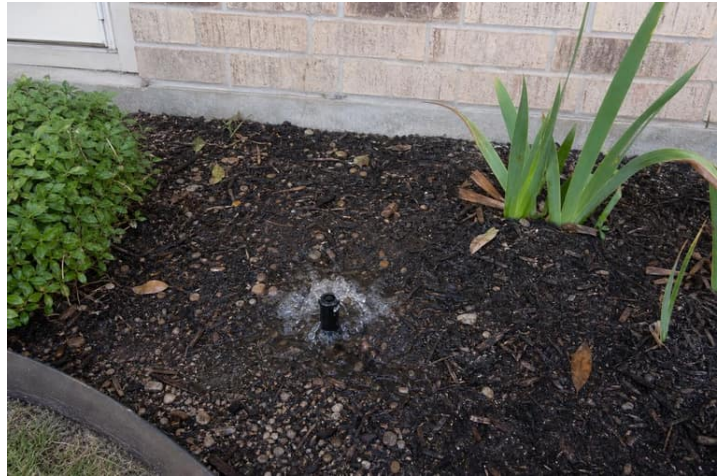
Sprinkler head bubbling from below grade during the manual zone test.
