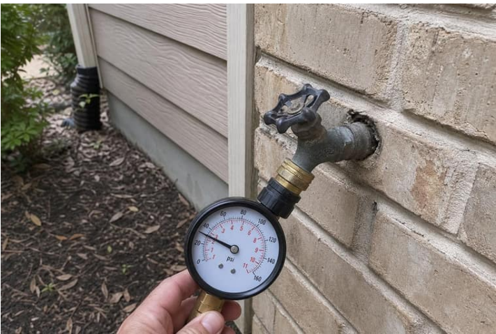
Static water pressure reading at an exterior hose bibb lacking anti-siphon protection.
