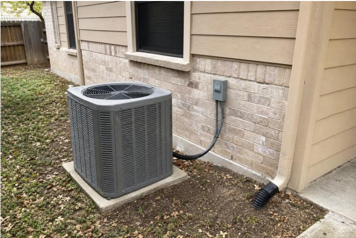
Heating equipment overview for the Texas REI QA report.
