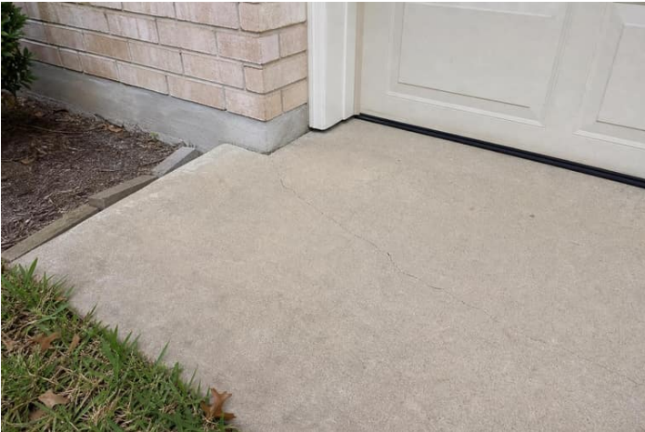
Minor hairline foundation cracking without significant displacement.
