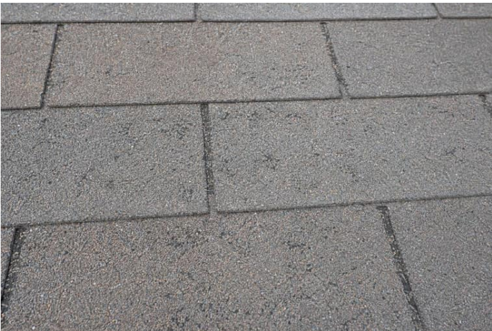
Localized shingle granule loss and surface wear.
