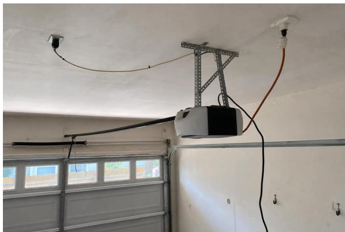
Garage door opener powered through an extension cord rather than a dedicated outlet.
