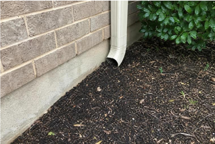
Downspout discharging near the foundation with limited clearance.
