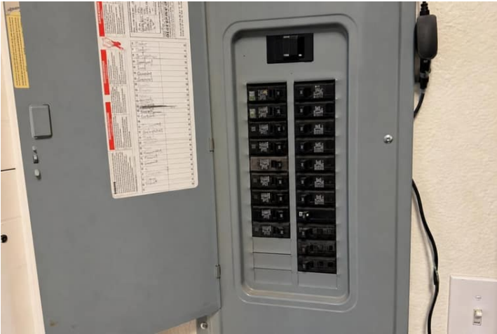
Electrical branch circuit concern with incomplete panel labeling.
