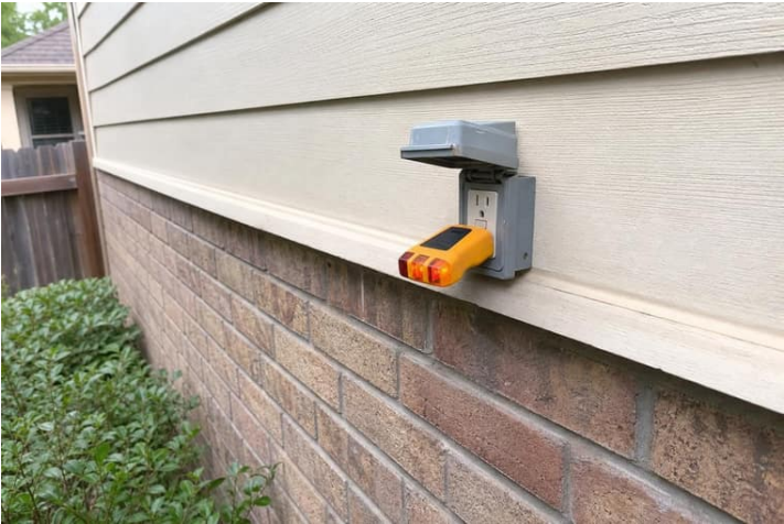
Exterior receptacle that did not respond to GFCI testing.
