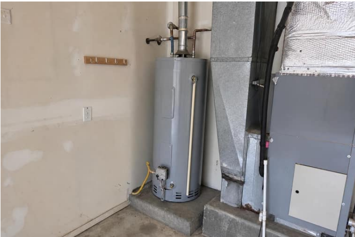
Natural-gas water heater overview with visible supply and venting connections.
