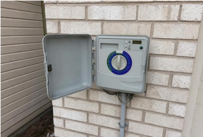
Irrigation controller with missing zone labels.
