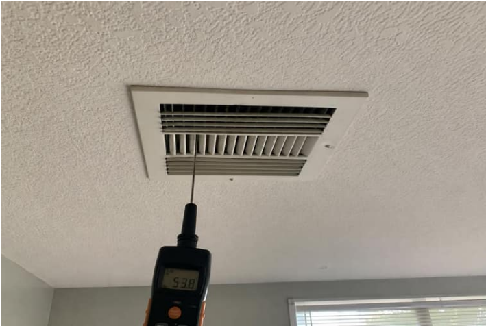
Supply register temperature check showing low cooling differential.
