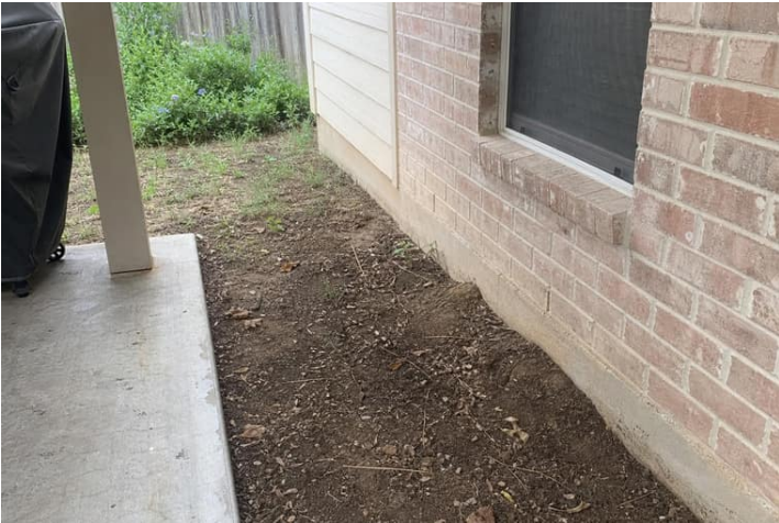
Soil contact and drainage clearance concern at the rear patio.
