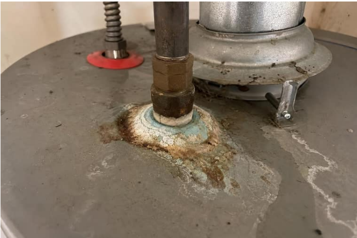
Corrosion and mineral staining at the cold-water supply connection.
