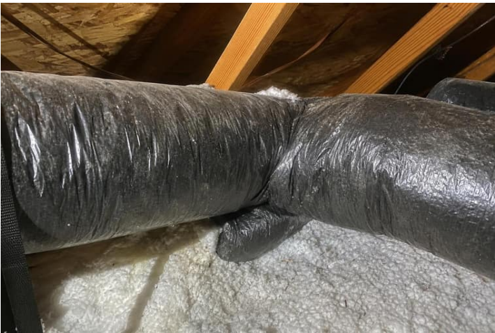
Flexible attic ducts in contact with compressed insulation at one branch.
