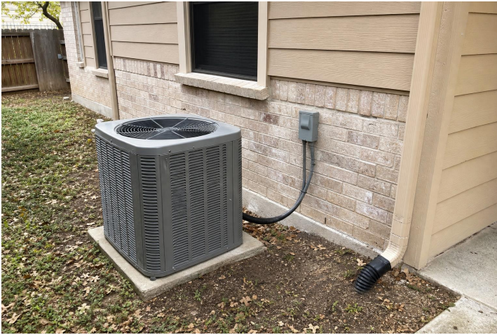
Heating and cooling equipment overview for the Texas REI QA report. - Heating and cooling equipment overview for the Texas REI QA report.
