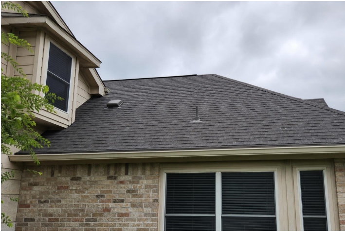
Composition shingle roof covering viewed from accessible ground and eave areas. - Composition shingle roof covering viewed from accessible ground and eave areas.
