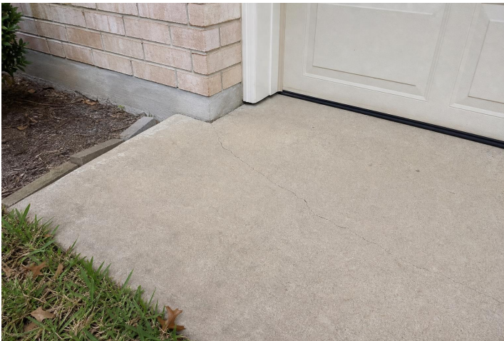
Minor hairline foundation cracking without significant displacement. - Minor hairline foundation cracking without significant displacement.
