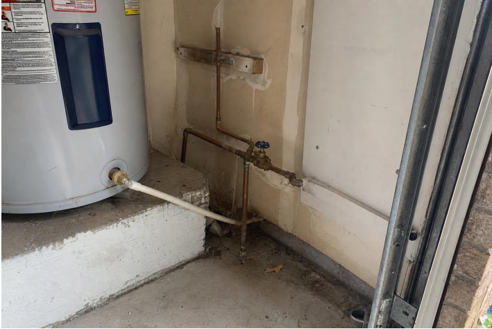
Main water supply valve and visible supply piping documentation. - Main water supply valve and visible supply piping documentation.
