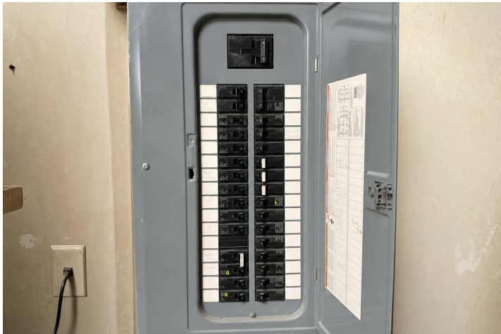
Electrical 7.5a - Electrical panel with incomplete breaker labeling.
