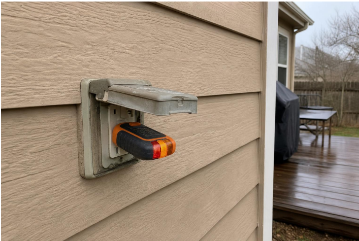
Electrical 7.9a - Exterior receptacle that did not trip during GFCI testing.
