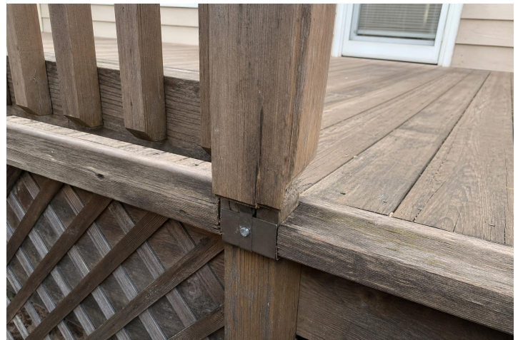
Exterior 2.8b - Closer view of guardrail post movement at the rear deck.
