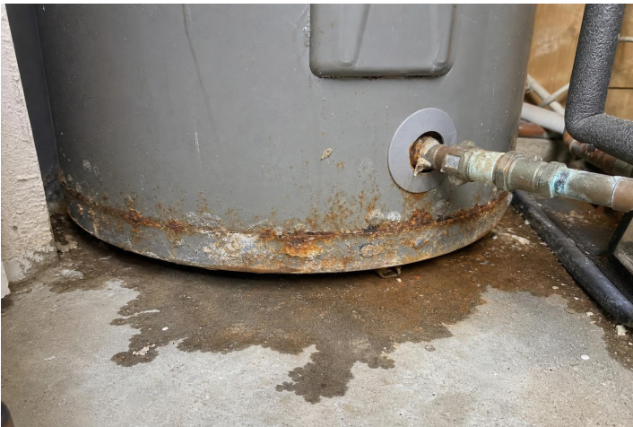
Plumbing 6.3a - Water heater corrosion visible near the lower jacket and connections.
