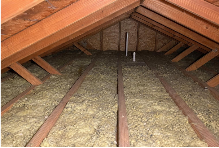
Attic, Insulation & Ventilation 9.1a - Attic insulation depth below modern energy-efficiency targets.
