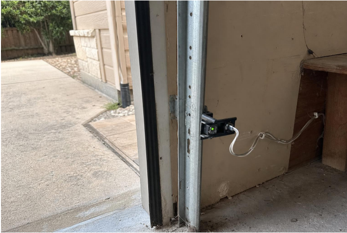
Doors, Windows & Interior 10.8a - Garage photo-eye sensors did not respond consistently when tested.
