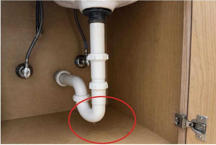
Plumbing 6.11a - Active plumbing leaks observed
