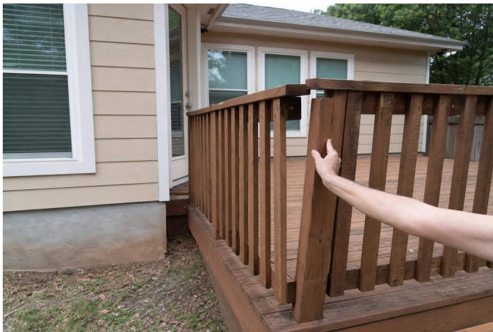
Exterior 2.8a - Rear deck guardrail at the loose east corner.
