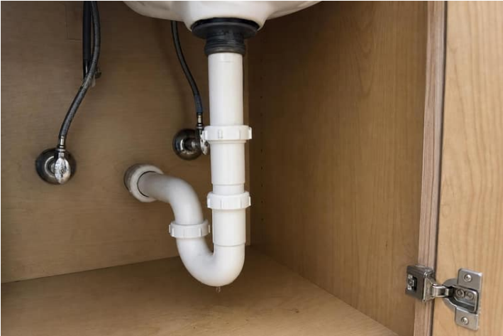
Plumbing 6.11a - Guest bathroom sink trap with active drip noted during operation.
