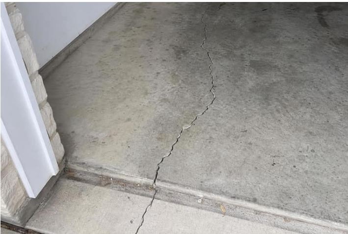
Basement, Foundation, Crawlspace & Structure 3.7a - Garage slab crack and minor differential movement indicator.
