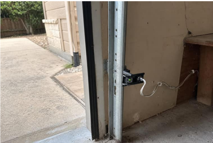
Doors, Windows & Interior 10.6a - Garage door photo-eye safety sensor concern.
